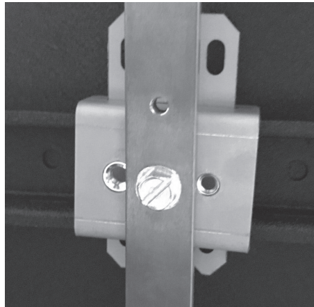
Copper Bus Grounding Bar
